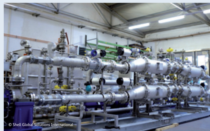
Nanofiltration membrane plant for desalination of oil-containing waste water
