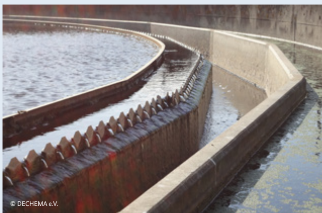
© DECHEMA e.V. Secondary clarifier of a waste water treatment plant
